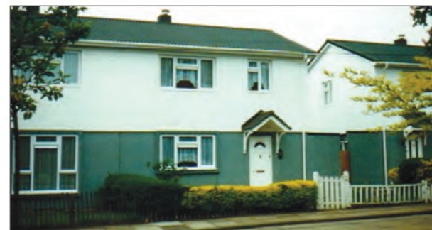
The Pantile 2000 fast-track roofing system considerably reduces time on site, keeping disturbance to a minimum.
