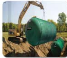
Rain Harvesting Tank
