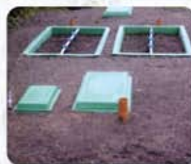
Treatment Unit With Sand Filters
