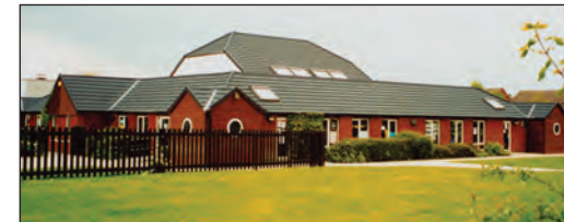
This school project used the 0.9mm thick Slate 2000 because of the high vandalism.
